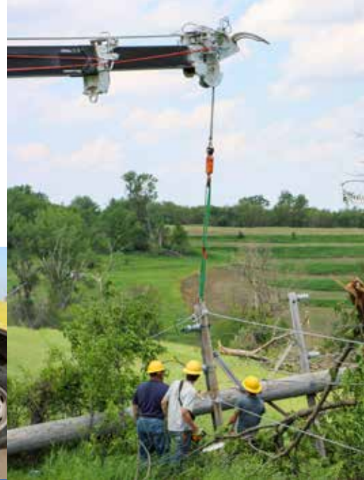
▶ Crews worked to lift a broken transmission pole in CIPCO's service territory.
