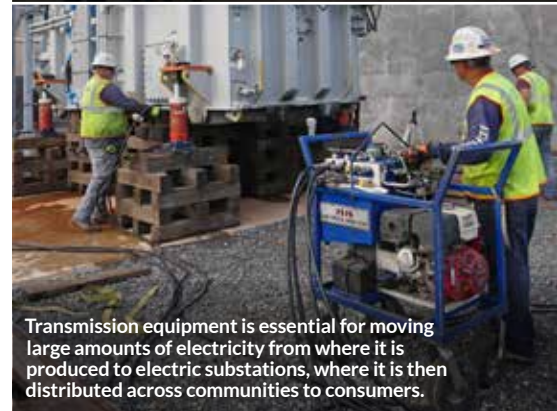
To keep pace with rising energy demand, new transmission equipment must be built, and existing equipment must be upgraded with the latest technology.
