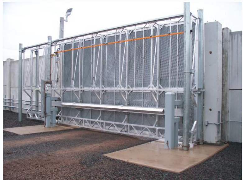
Right: PPL Electric Utilities, TCGR-12.
