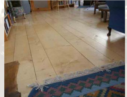
Sycamore floor, 24mm boards up to 400mm wide, which after 5 years show max 5mm gaps between. These may need to be filled, or boards moved.
