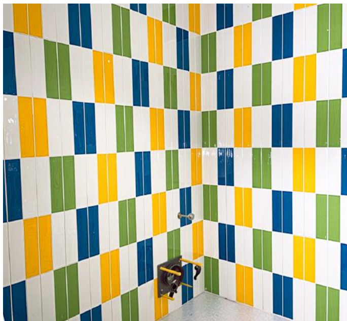
Hulme used LATICRETE MULTIMAX™ thinset and SPECTRALOCK® grout in a school to install this boy's bathroom.
