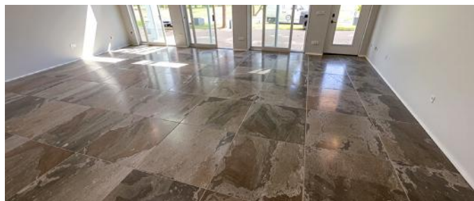
This 36" x 36" flooring was installed over a hydronic heating system, using Schluter-DITRA® and thinset and MAPEI grout.
