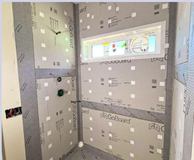
Sean Wahl, tile contractor in Omaha, Neb., installed these GoBoard Membrane products.
