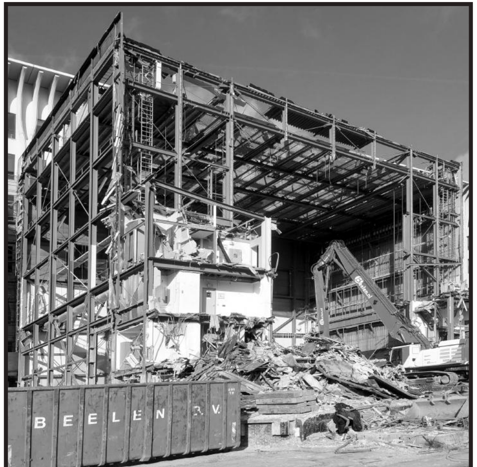
The stage-house of the Lucent Danstheater being demolished in January 2022. NDT's new home, Amare, can be seen behind it. Photo by Michael Hasted
