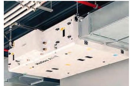
A total of 75 Helios Air1 XC ventilation units are being installed across the three sites
