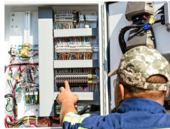
Easy Access to Heavy Duty Circuit Breaker Panel and Breaker Reset Switches
