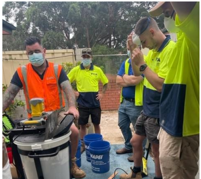
Jim and Will from Mapei teach the eager apprentices the correct process
