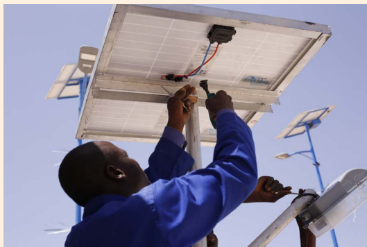
Niger youth gaining skills on installing and maintaining newly installed solar panels. UNDP Niger.
