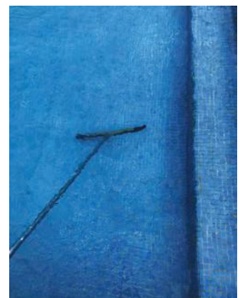
Check the grout in tiled pools
