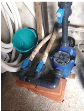
Look out for bad pump installation
