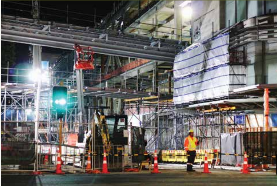
Undergoing maintenance is a dedicated activity
