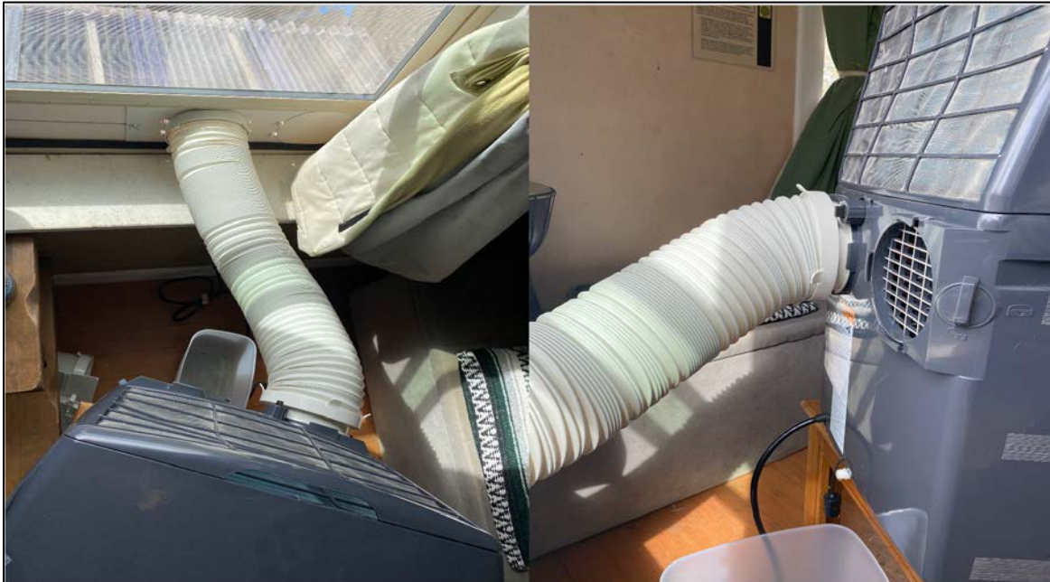
Figure 4: Back view of the Haier unit showing the dual exhaust system connection and the water bucket installed for condensation to drain in. The heat pump does not come with a water pump that could pump the water outside, so only gravity was used. The second hose was not used in this case because the indoor air was cold and sufficient enough to cool the compressor during heating mode.
