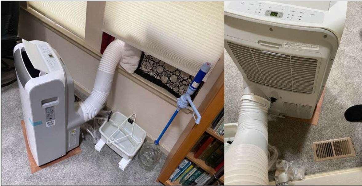
Figure 3: Back view of the Whynter unit showing the single exhaust system connection and the water bucket installed for condensation to drain in. The heat pump comes with a water pump that could pump the water outside, but the homeowner preferred using gravity and emptying the bucket often than sending the water out using the pipe and causing a possible air leak into the house.
