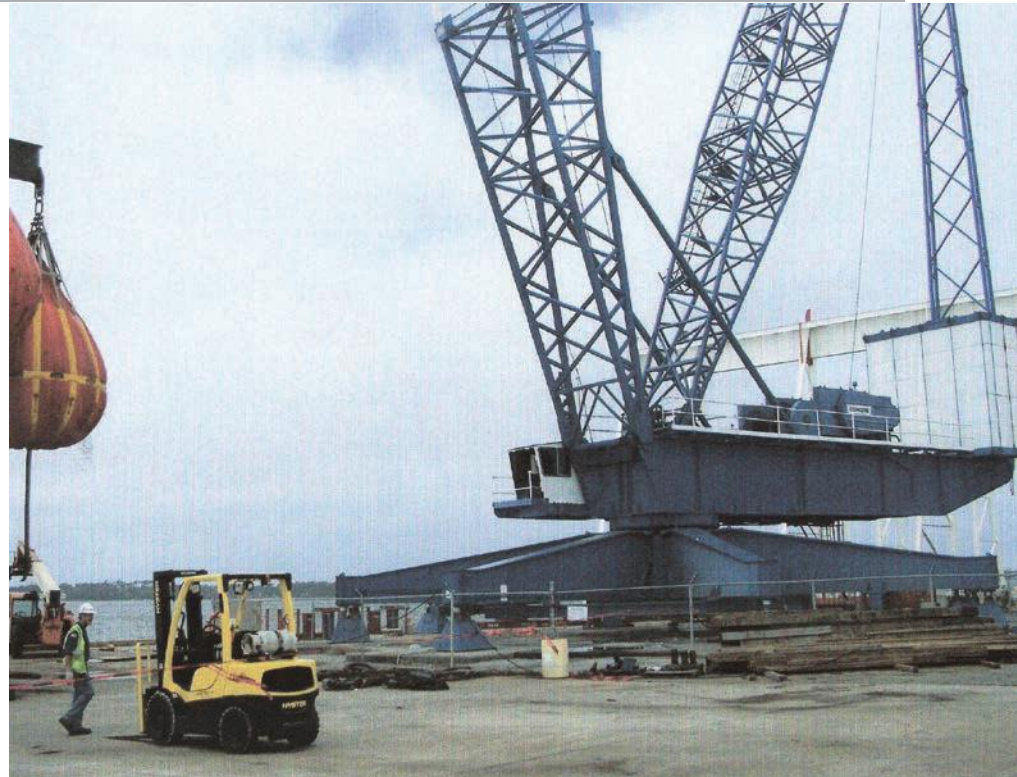
Fig. 1. Heavy-lift cranes are often leased for up to five years for plant construction.
