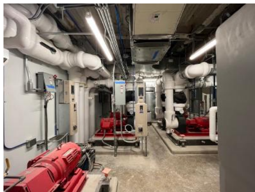
Updated mechanical systems in the boiler room.
