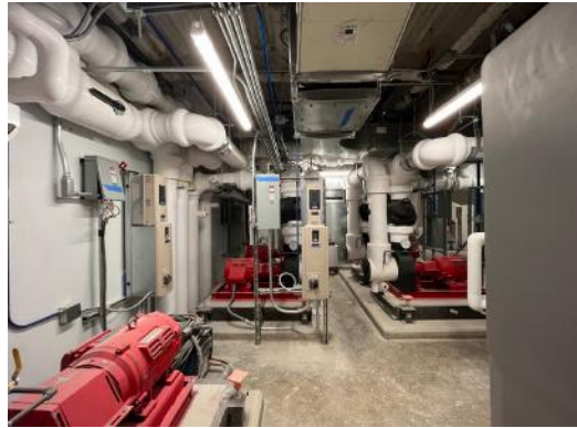
Updated mechanical systems in the boiler room.
