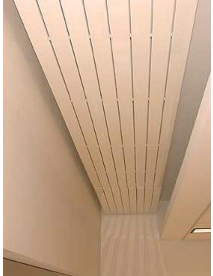
Radiant ceiling panels installed linearly show they are both a utility and architectural feature.
