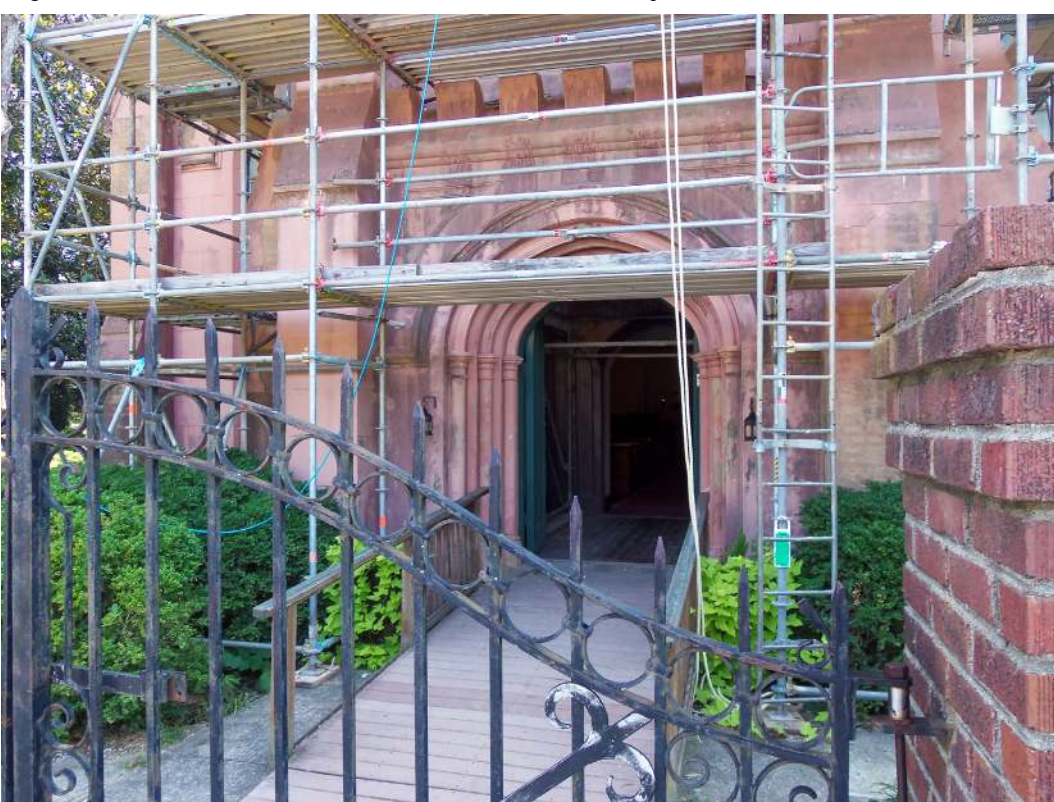
Trinity Episcopal Church is still in the process of being restored, as can be seen here. The Abbeville church is considered a fine example of Gothic Revival architecture. (Staff photo by Henry E. Green)
