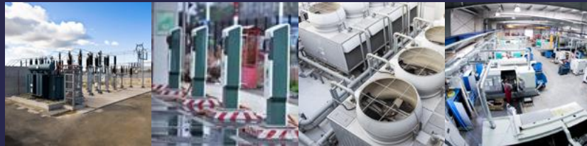
Substations Charging Stations Chemical Plants Industrial Laundries
