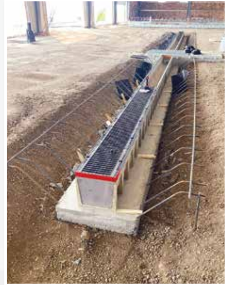
Trench drain system for the RM of Buckland Maintenance Shop. CT Distributors Inc.
