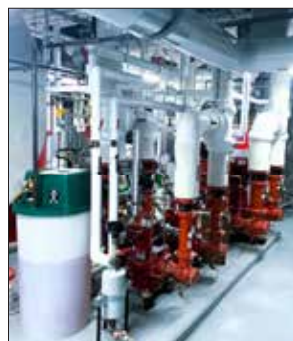
West Coulee Station Elementary School Mechanical Room
