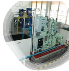
PURIFIER FRESHWATER GENERATOR OILY WATER SEPARATOR
