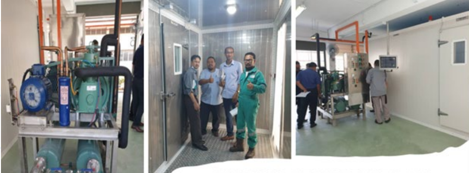
MARINE REFRIGERATOR & COLD ROOM
