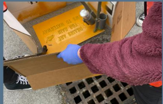
Responded to over 5,000 OUPS tickets to mark locations of water, sanitary and drainage lines.
