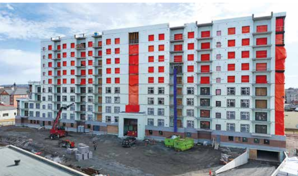
The Railyards is designed as a rental community, not a condominium project, and fits Colpitts's long-standing model.
