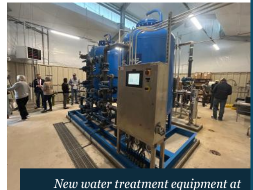
New water treatment equipment at Louviers Water and Sanitation District.
