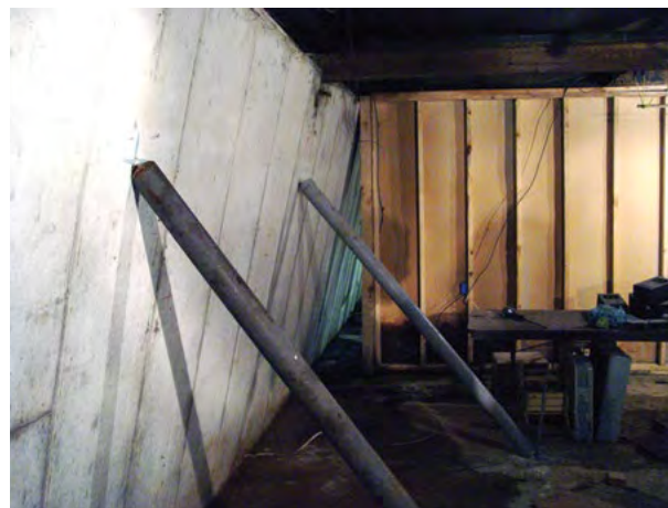
Figure 3.2 Poured concrete walls often lean in at the top and show less cracking in the interior portions of the wall
