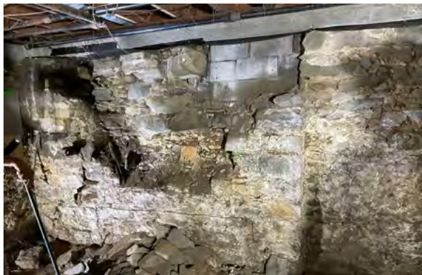
Figure 3.5 Before: Severely damaged CMU block wall
