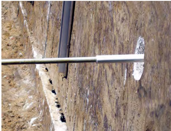
Figure 3.13 Before: Shear movement of a block wall evident from exterior
