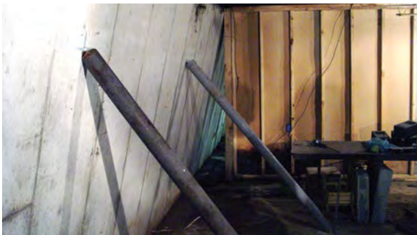
Figure 3.11 Before: Poured concrete basement wall severely leaning in at the top
