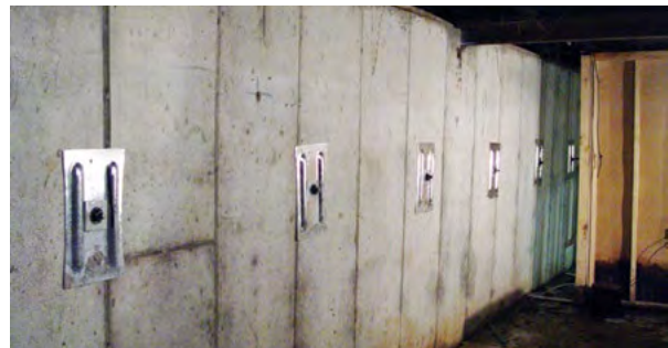
Figure 3.12 After: Wall is immediately returned to original straight position after backfill soil is removed and GeoLock anchors installed
