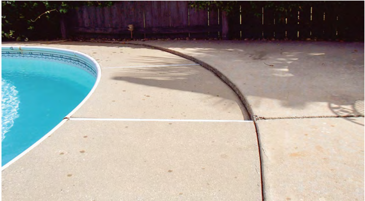
Figure 5.5 Pool deck slab settlement
