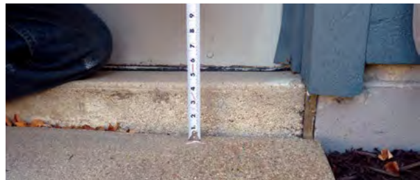
Figure 5.3 Before: Driveway settled up to 4 inches relative to garage slab
