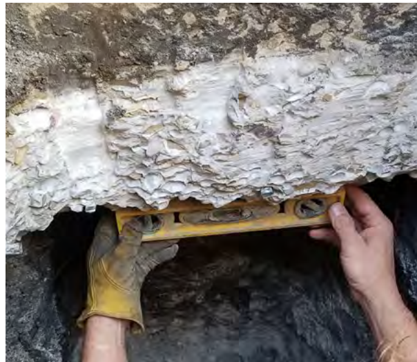
Figure 2.48 Prepare bottom of footing with chipping hammer, as necessary, to create a flat and level surface
