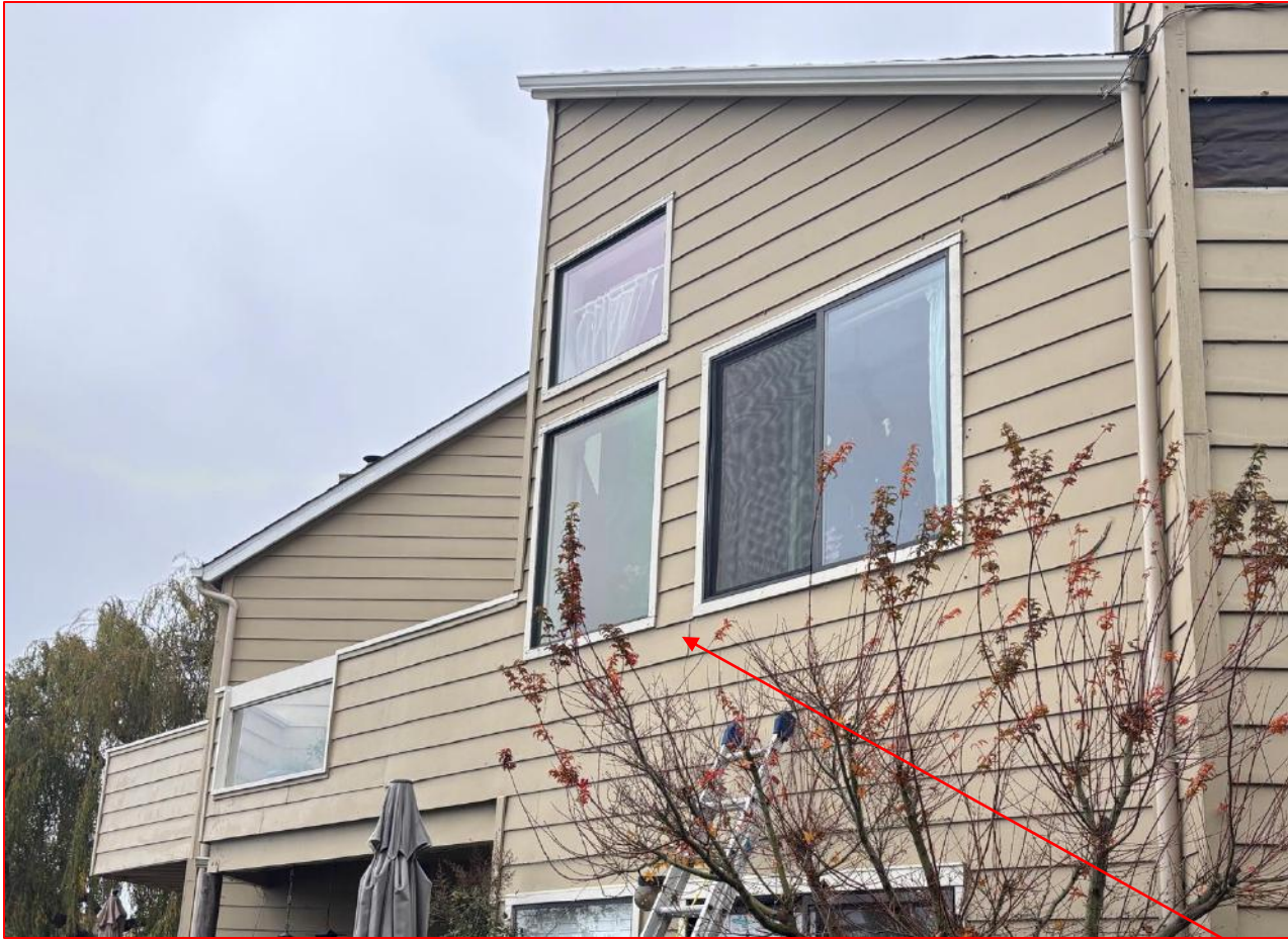
Typical Updated Flanged Window Installation, Aged WRB, and Existing Flashing Sequences. Noted Felt Paper WRB, Jamb Flashing, and Sill Flashing
