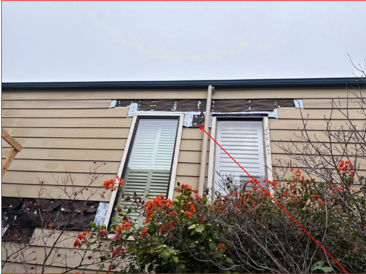
Updated "Spot" repaired WRB, Window flashing, and original aged and worn Felt Paper WRB
