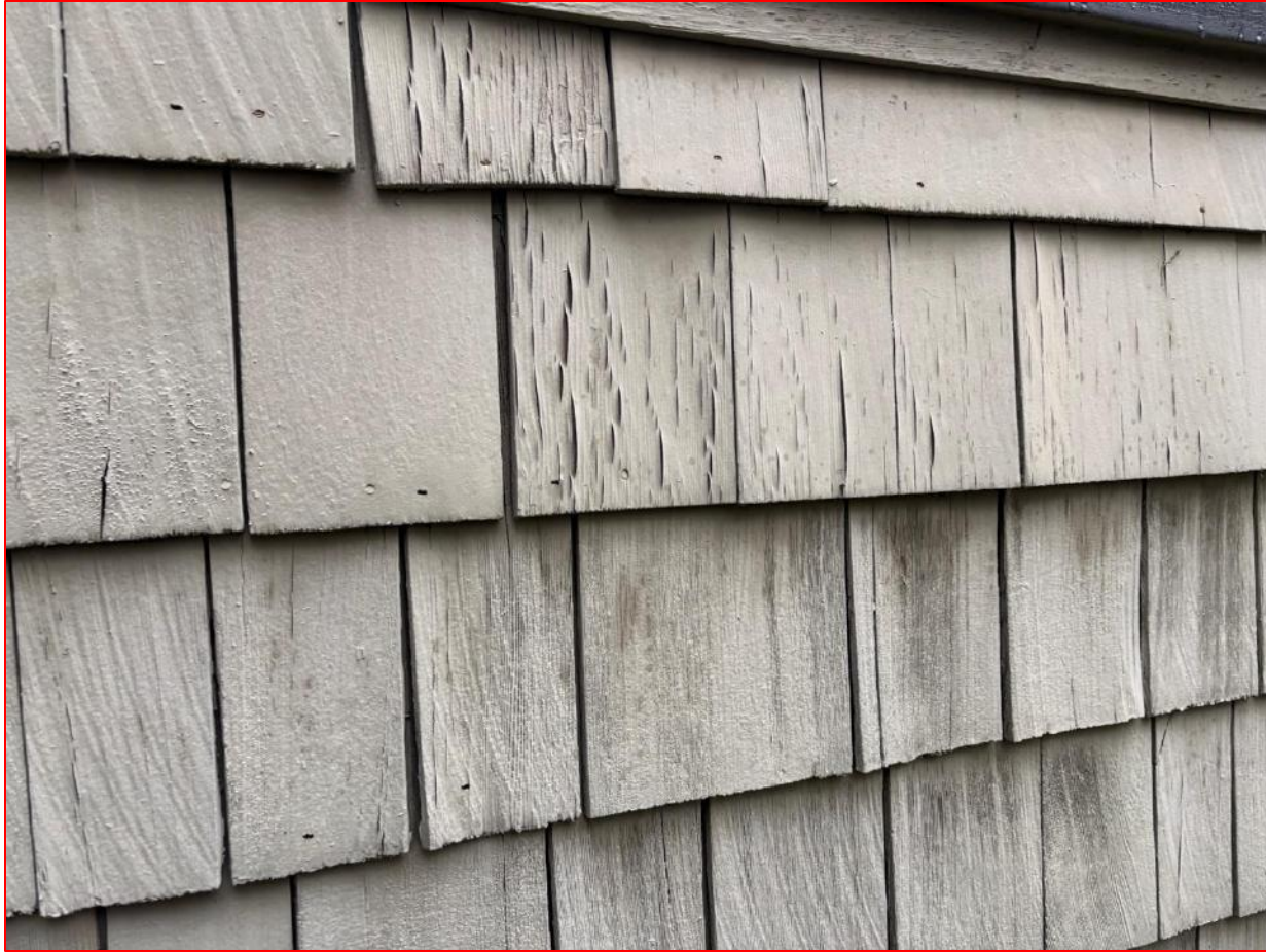
Adhesion and Coating Failures - Pervasive
