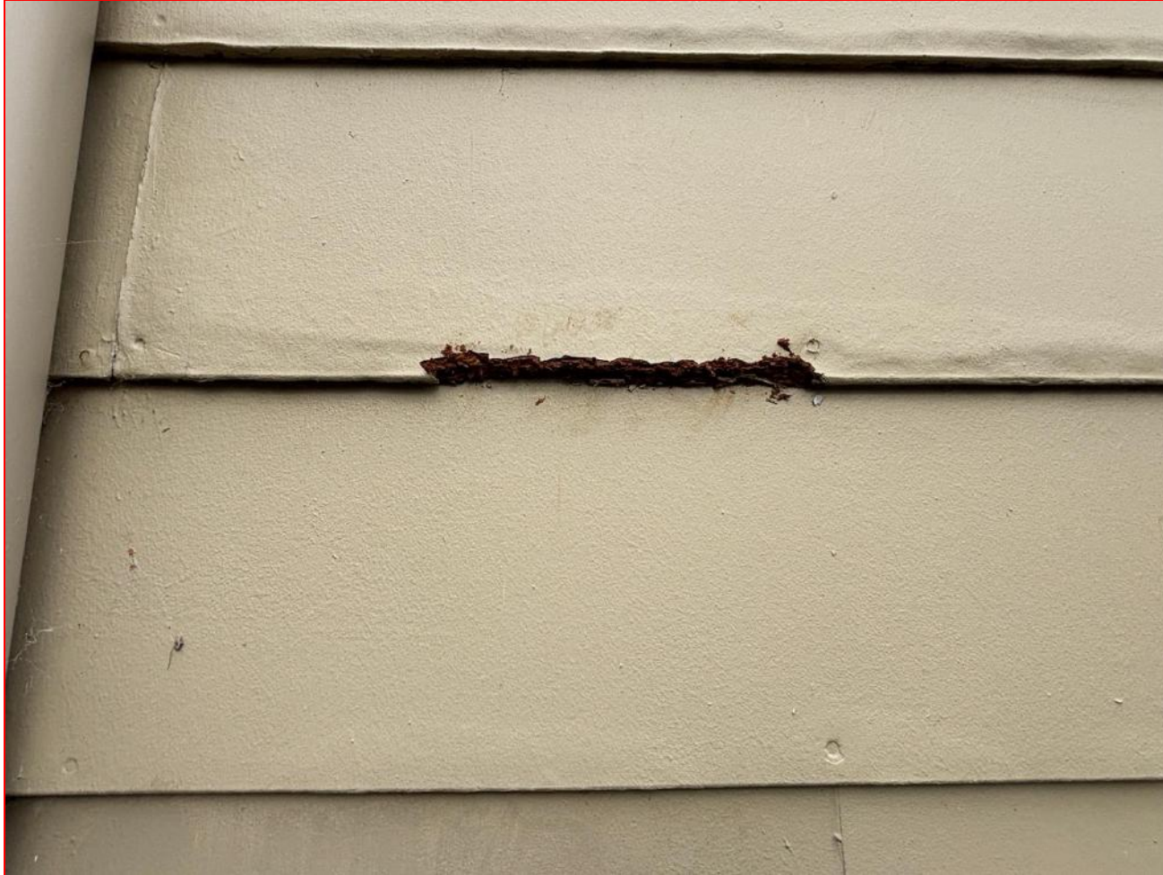
Noted moisture-damaged and deteriorated lap siding - Pervasive
