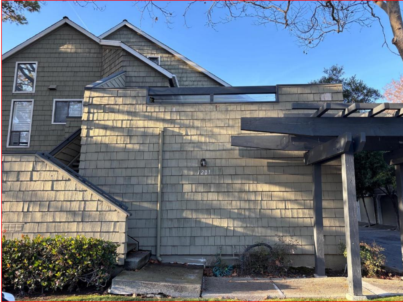
Cupped, Curled, and Decayed Wood Shingles - Pervasive
