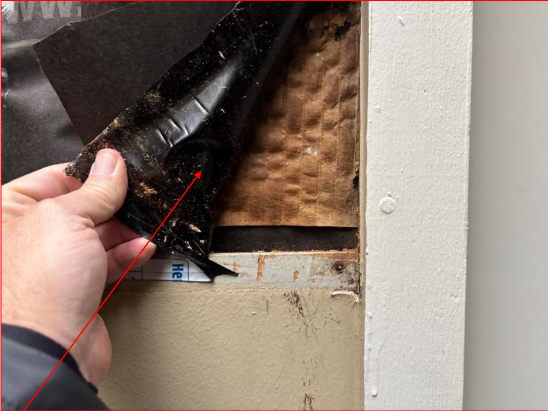
Noted updated “Spot” repaired lap siding, trim, membrane flashing, and WRB – Noted additional sealant added to WRB fastener heads.
