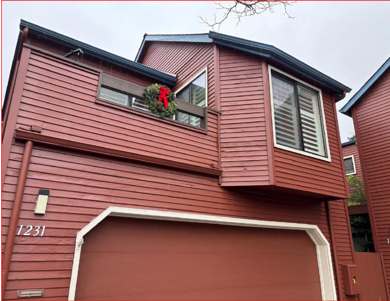
Aged, Worn, and Decayed Wood Siding Surfaces - Pervasive
