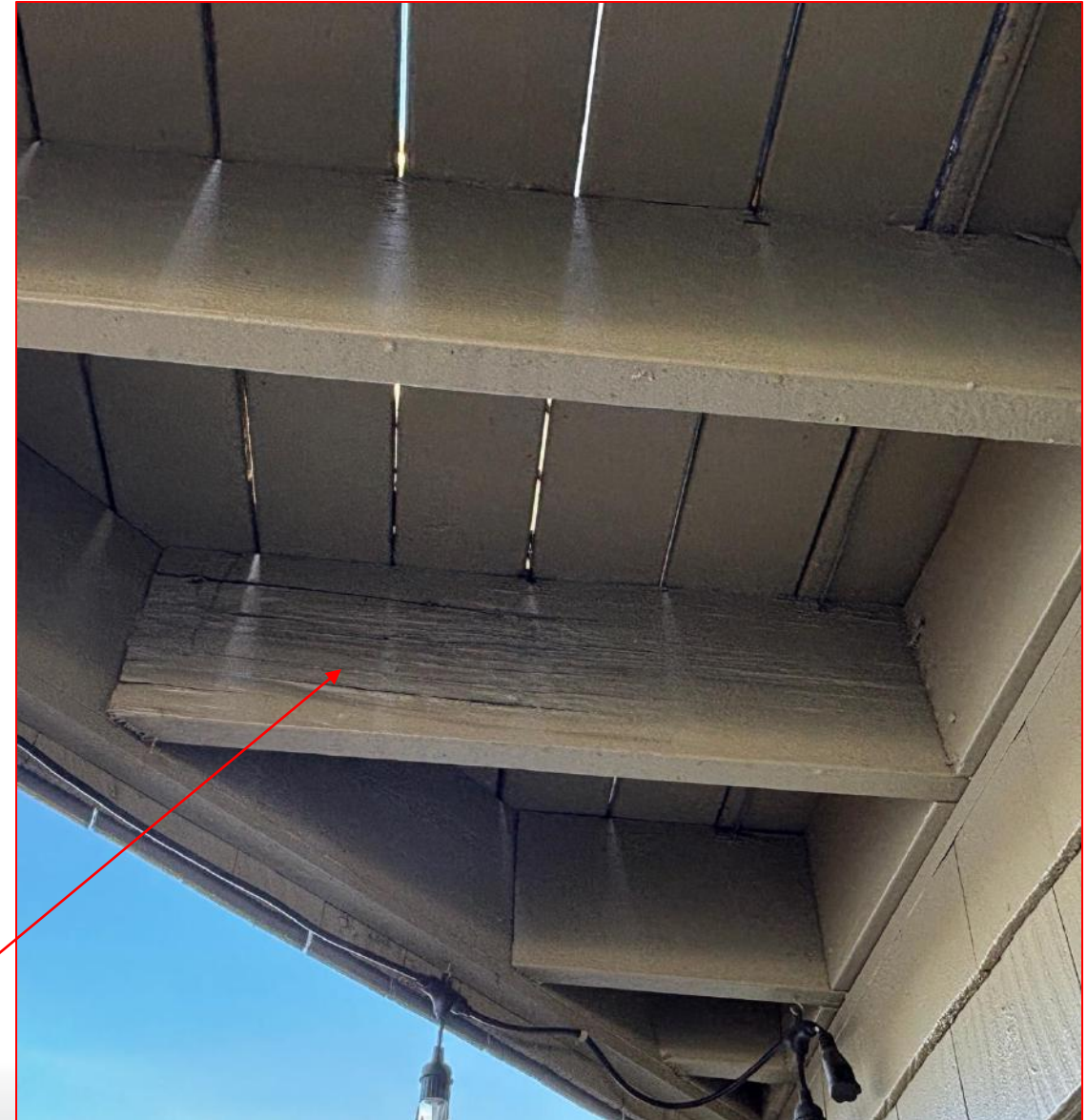
Visible framing decay, damage, and rot on wood cantilevered balconies.
