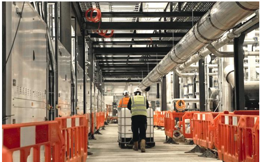
Preparing to charge the heat pump system with Thermox DTX Picture credit: Oasthouse Ventures
