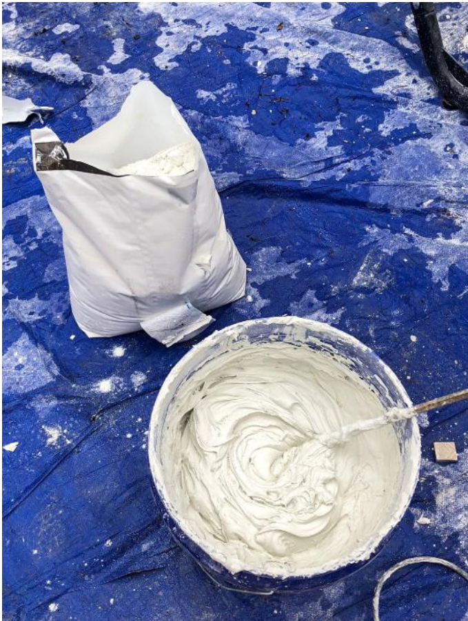
Mixing is one of the first steps in the installation process, and it sets the stage for everything that follows. Follow the mortar manufacturer's mixing speed instructions!
