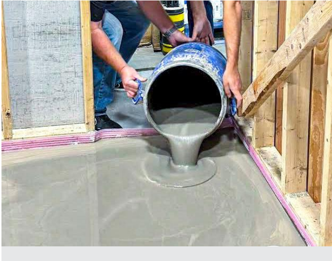
At another NTCA Regional Training program, self-leveling compound is poured to attain floor flatness
