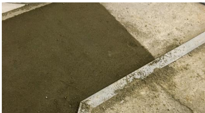
Installers at Welch Tile used a mortar bed to achieve the desired floor flatness.
