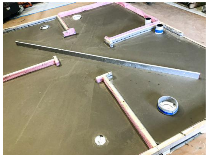
At a 2021 NTCA Regional Training program held at D.W. Sanders Tile & Stone Contracting, a 10' straightedge is used on a flat floor achieved by a self-leveler.
