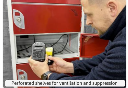
Linear heat detection cable in each compartment for early fire detection
