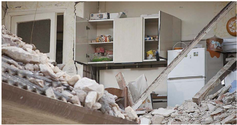
Significant damage to a house following an earthquake. Photo: Pixabay.com.
