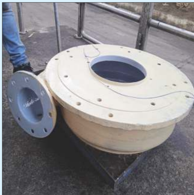
The steam cooker was ready to be put back into service after the 24-hour curing period.
