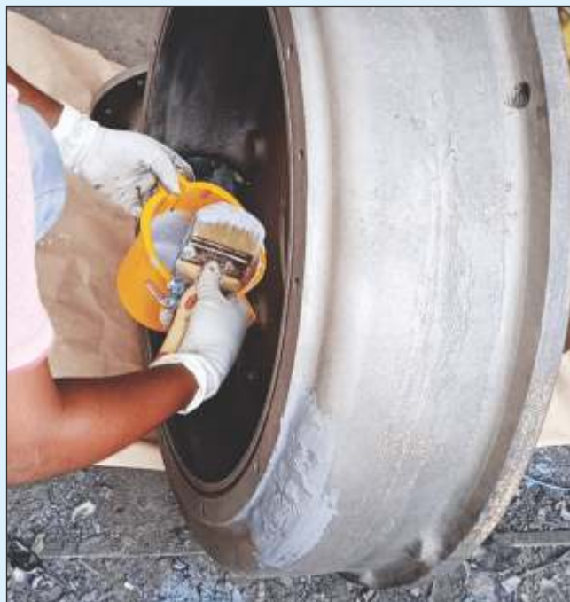
An initial layer was applied with a brush, followed by rebuilding with more product using a Belzona applicator to restore the surface to its original profile.
