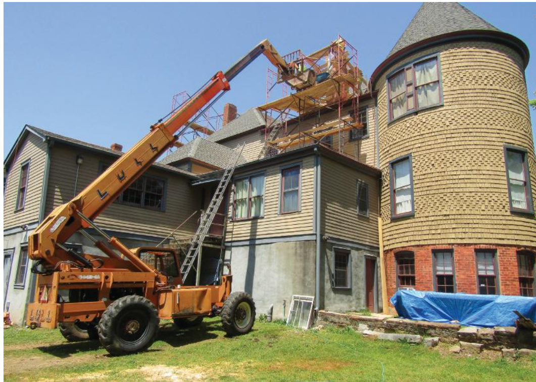
This Abbeville County Historical Society is working with K and D Contracting Services of Columbia to stabilize a chimney on the roof of the Society's McGowan-Barksdale-Bundy House in Abbeville. (Staff photo by Henry E. Green)
