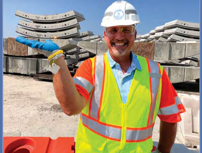
Cape Charles Mayor Adam Charney visits the project to see how the tunnel segments manufactured in Cape Charles are placed by the TBM.
