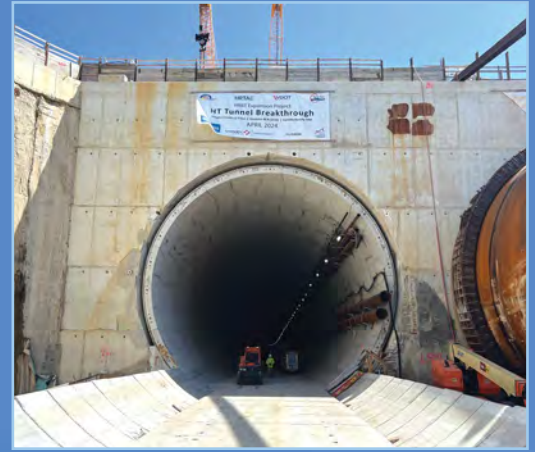
[ABOVE]: After the breakthrough, crews work inside the tunnel to make way for the new road.
