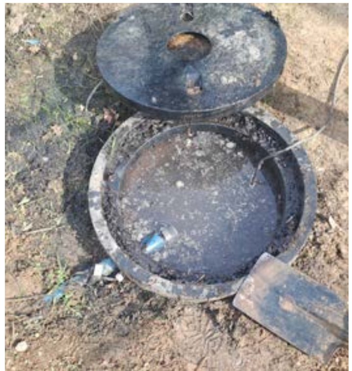
Figure 4 A manhole at one of the study participants' wastewater treatment facilities
