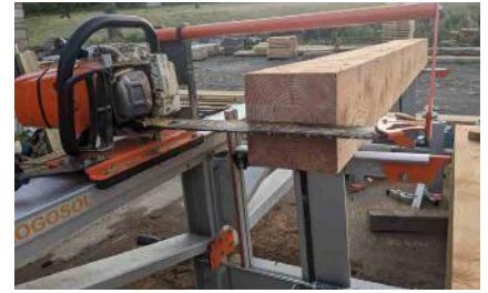
- A novel job for the Logosol F2 chainsaw mill - cutting slots into posts for the Dobie's house building project, to fit them onto the post bases. It was quick, accurate, and straight-forward. As well as being used in the sawmill (as the photos show), it was also easily carried up to the house-site and set up there to do the process in-situ.
