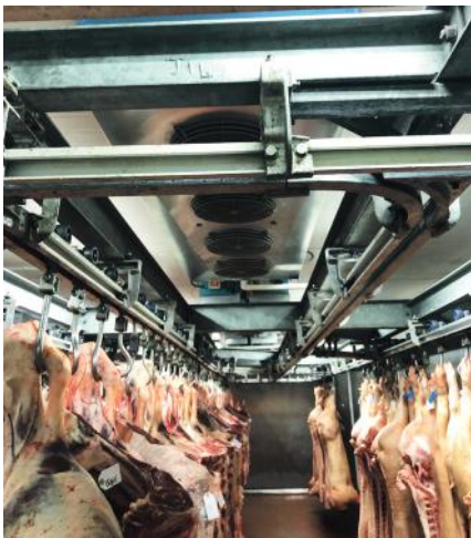
The units cool the meat store, which is maintained at 1°C
