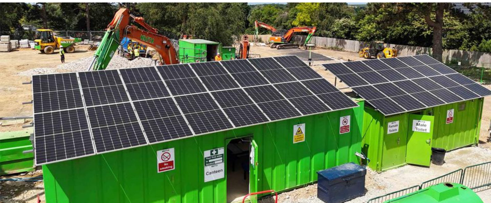
Solar PV Panels & Wind Turbine at our Sittingbourne Project
