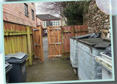
John St/West King Street – before & after of bin Store
