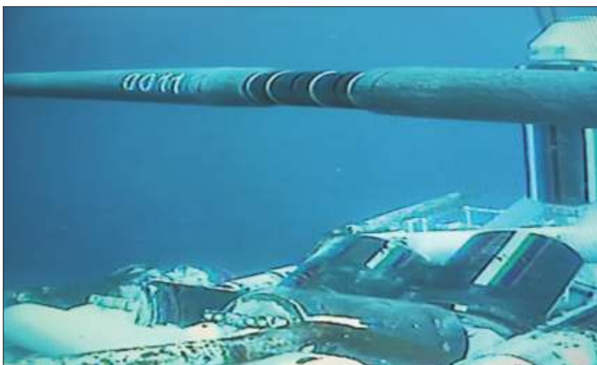
The completed Viscotaq Offshore Field Joint Coating (OFJC) system once deployed into the water.
