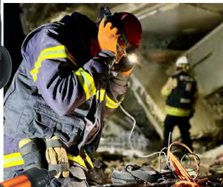
Above: It's been a bad year for earthquake fatalities largely due to the Turkish 'quake killing almost 60,000 but Afghanistan and Morocco also saw almost 3,000 deaths each. This picture shows Leader Group's acoustic listening system deployed in Turkey p2-4 and we discuss drone use on p18
