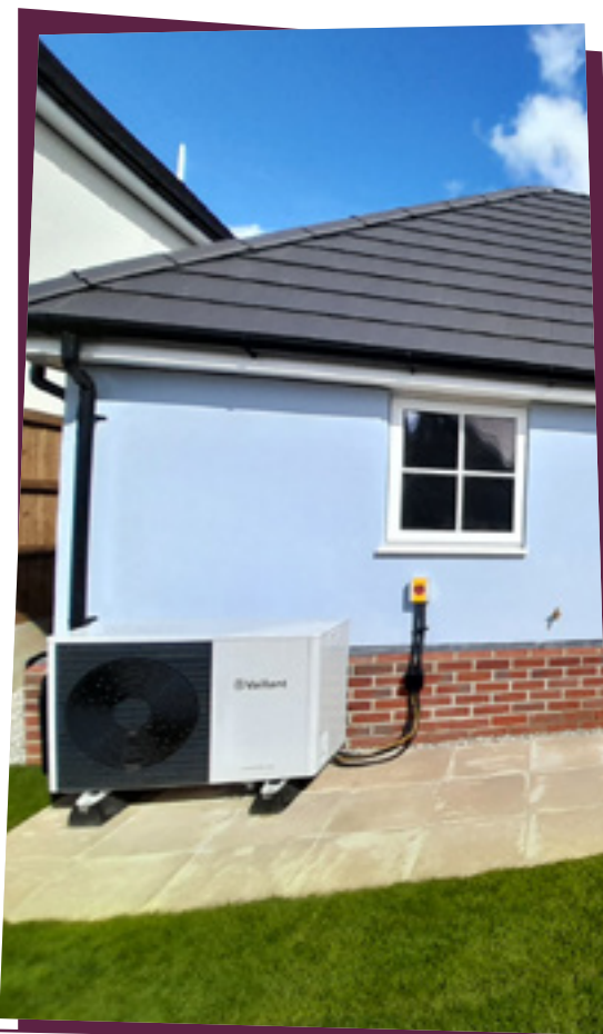
An ASHP on a new home
