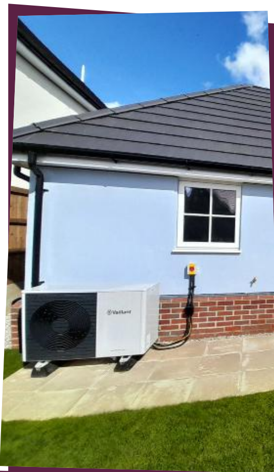
An ASHP on a new home
