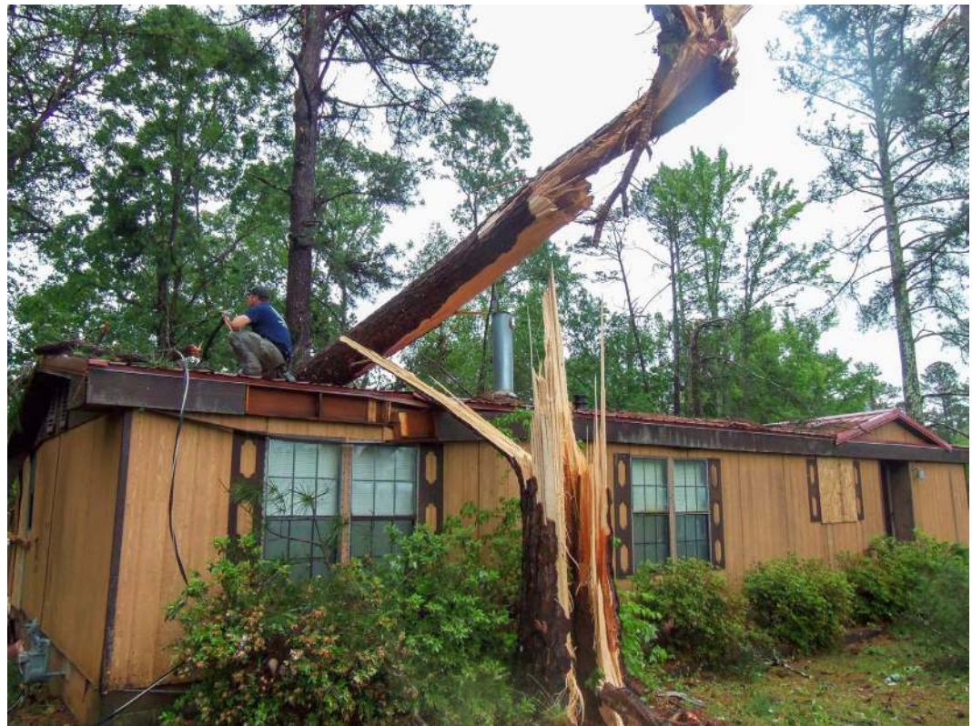
This home on the eastern outskirts of Abbeville was one of the homes damaged during a storm Monday afternoon, as the County was under a tornado warning for much of the afternoon. (Staff photo by Henry E. Green)
