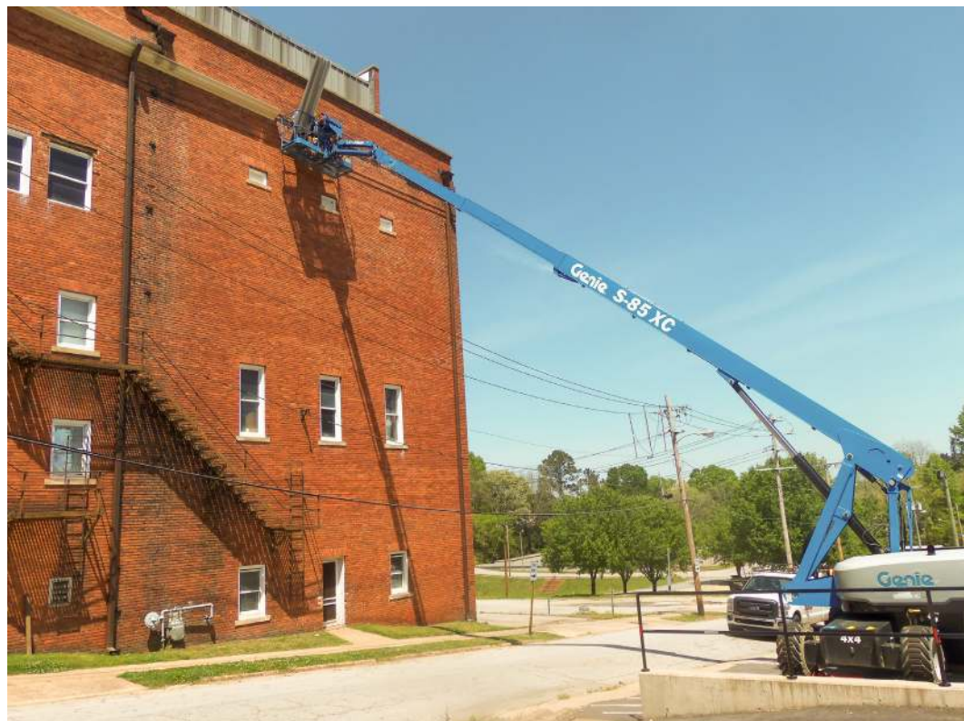
Lloyd Roofing recently could be spotted doing some work on the exterior of the Abbeville Opera House. Here is a bucket truck putting some finishing touches on a wall facing East Pickens Street. (Staff photo by Henry E. Green)
