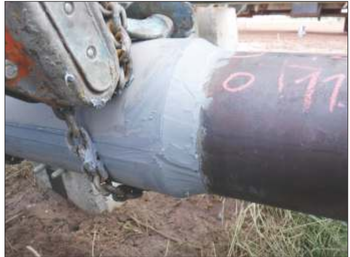
The plates were held in place by a fixed hoist to allow the product to cure.
