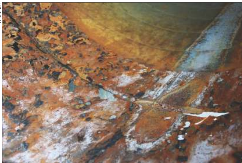
Internal corrosion can eventually result in leakage, cracks, and rupture of the pipeline leading to explosion hazards and methane emissions.
