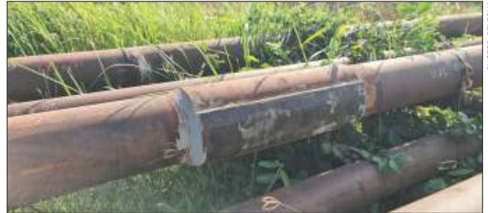
The pipeline was exposed to corrosion at the joints where sections had previously been welded together.
