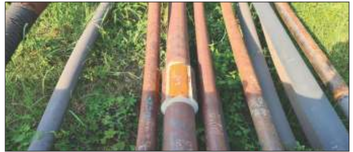
Belzona's cold bonding solutions had previously repaired other areas of the pipeline.
