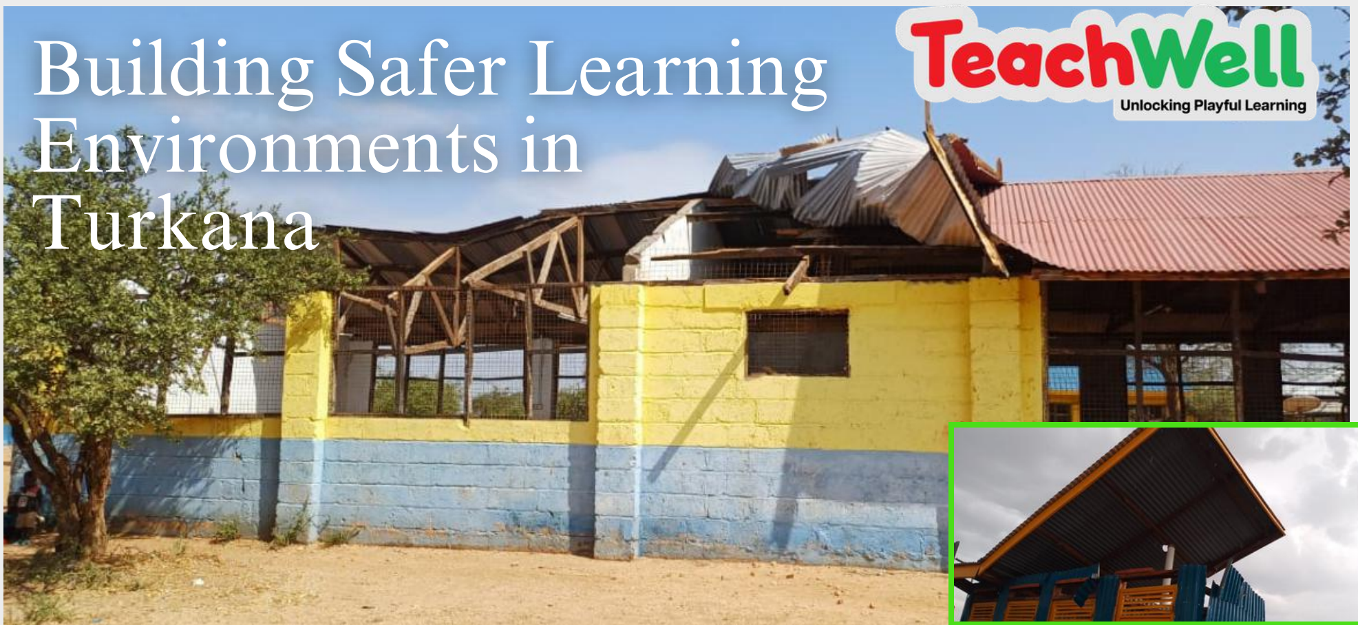
Roof blown off a classroom block at Korinyang Primary School in Turkana South. Photo: Vincent Mageto / IRC.
