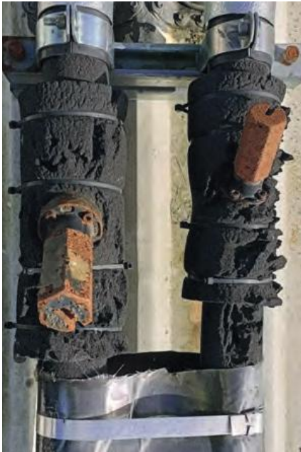
Insulation should be considered as a system. How is the insulation secured? Is there a vapour seal at fixing points?
