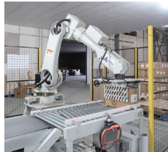
An industrial robot installed for palletizing finished products.
