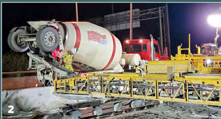
[ABOVE 1]: Crews inspect the rebar support where the original Willoughby Bay Bridge will be connected to the newly widened section.
