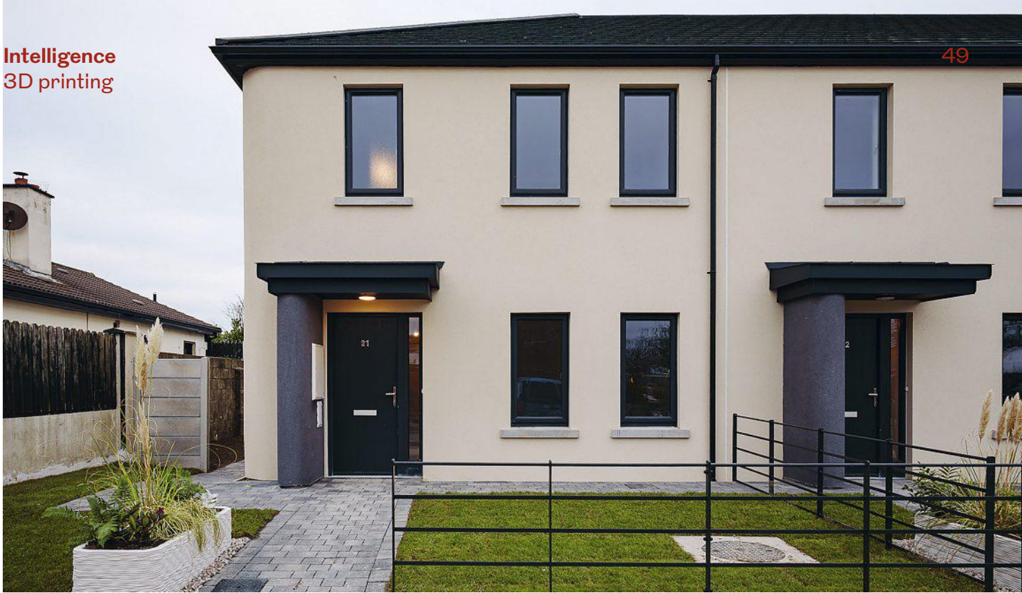
Above The three social homes printed by COBOD's BOD2 machine are the first to meet a new ISO standard for 3D-printed construction.
