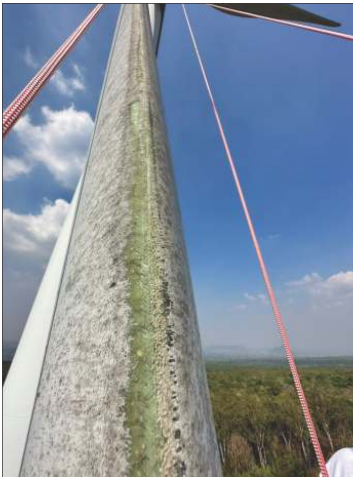
Leading edge damaged by erosion.
