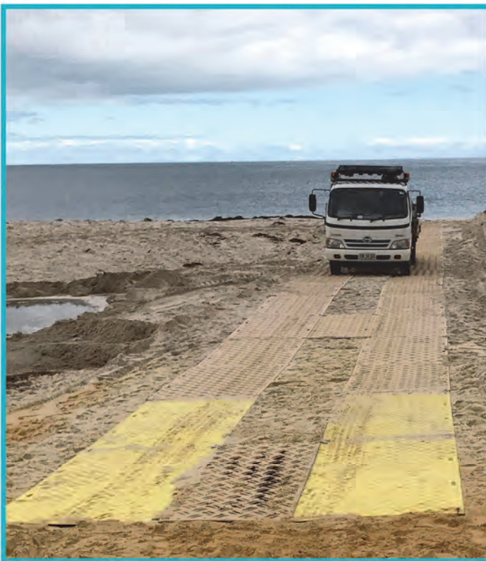
Beach access mats are installed at Normanville Beach ready for the summer season
